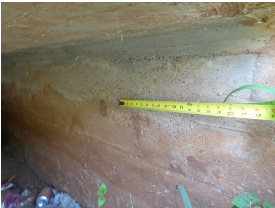
Photo 22: Scaling occurring along the top 12" of the culvert walls, typical
