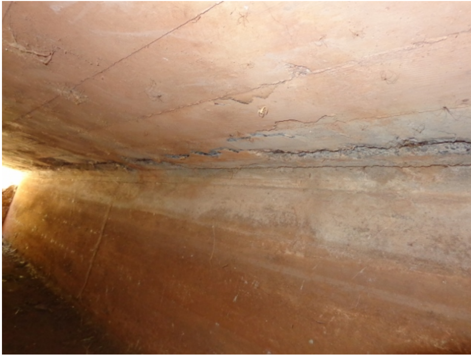
Photo 19: Spall measuring 10' long x 24" wide x 2" deep with 8 exposed reinforcing bars occurring in culvert soffit near outlet above the west culvert wall
