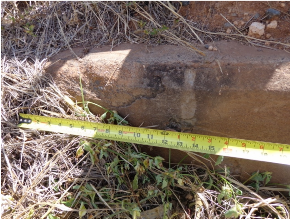
Photo 15: Spall measuring 8" high x 16" wide x 1" deep occurring at the top east corner of the upstream headwall
