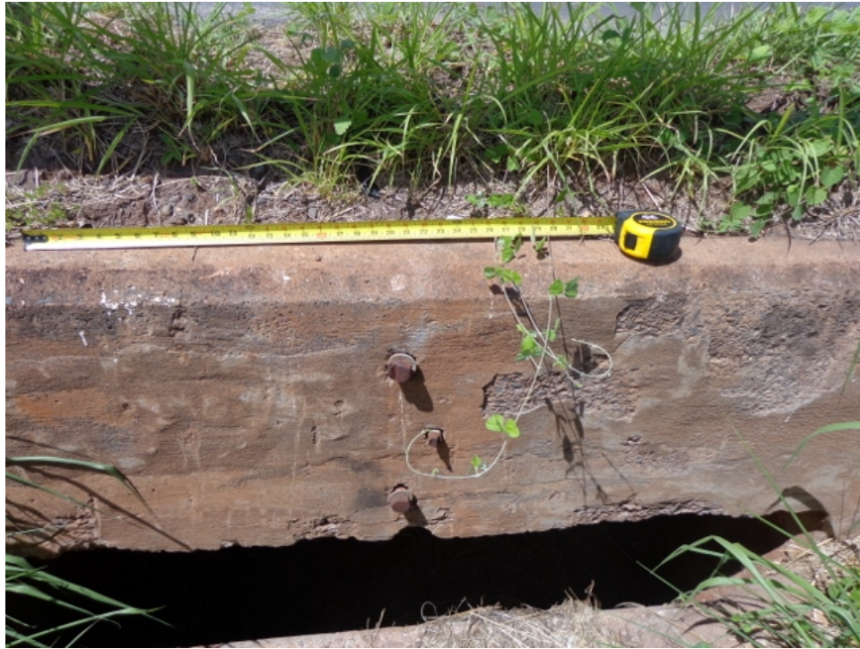
Photo 25: Scattered spalls occurring throughout downstream headwall
