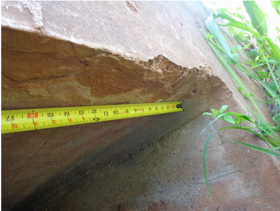
Photo 17: 12" long x 72" wide area of delamination occurring in culvert soffit at inlet
