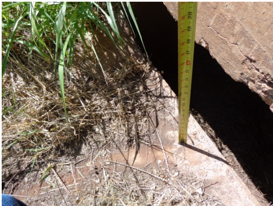
Photo 26: Concrete block built at outlet leaves only the top 16" of the culvert for water to flow through
