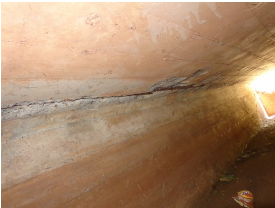
Photo 18: Spall measuring 10' long x 30" wide x 2" deep with 8 exposed reinforcing bars occurring in culvert soffit near outlet above the east culvert wall
