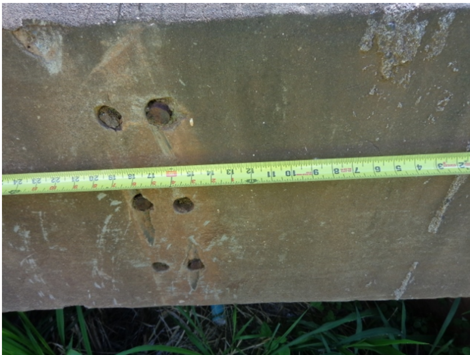
Photo 14: Corroded upstream guardrail posts embedments in upstream headwall
